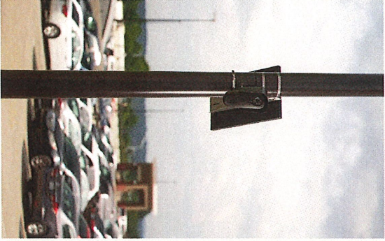
Solar & Existing Pole
