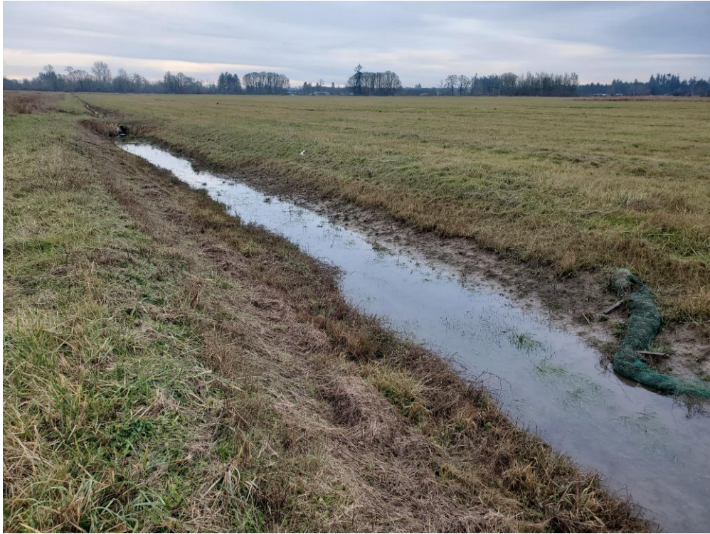
Existing irrigation ditch running east-west on the northern portion of the site.
