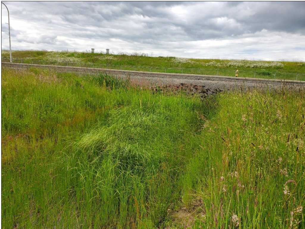
Figure 19. Drainage ditch and culvert under Rush Road near probe #16. View to the west-southwest.
