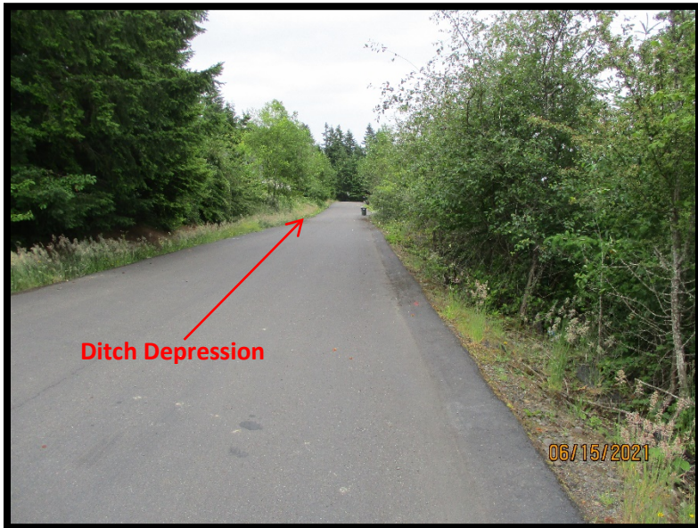
Photograph 3: Looking east along Hosanna Lane with subject site to the right. The V-shaped ditch to the left has a prominent depression opposite the garbage can where water ponds and seeps under the road from left to right onto the subject site.
