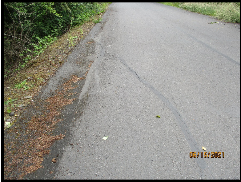
Photograph 4: Settling cracks on Hosanna Lane from saturated conditions under the asphalt. The subject site is to the left and ponded V-shaped ditch to the left.
