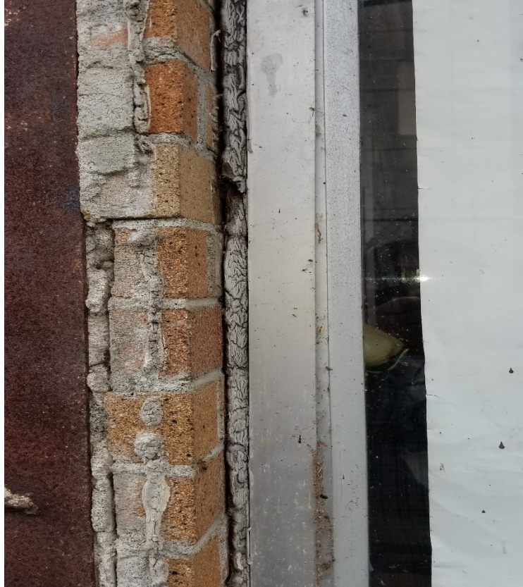
Exterior ACM window frame caulk. Northeast corner of building at Rec. Manager's Office
