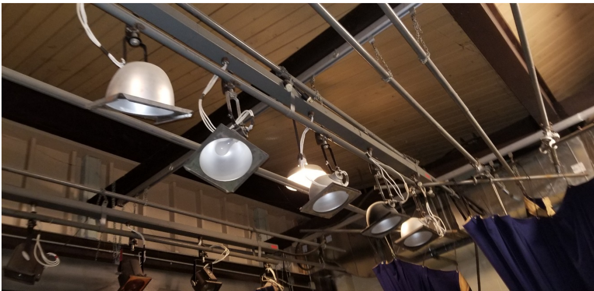
Presumed ACM white insulation on stage light wiring.
