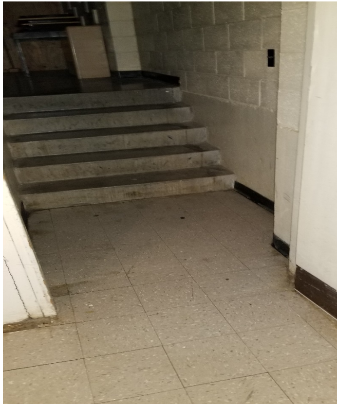
Typical 9" Light Brown vinyl tile. The mastic is non-ACM. Lobby of Restroom SE off Gym, Rm 108 – 111, Rm 114, Rm 116, & Rm 117
