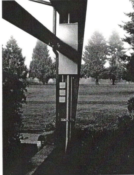
Elec Box – left side building
