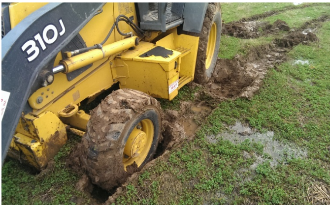
Photo 4. Excavation Equipment stuck in Soft Surficial Soil
