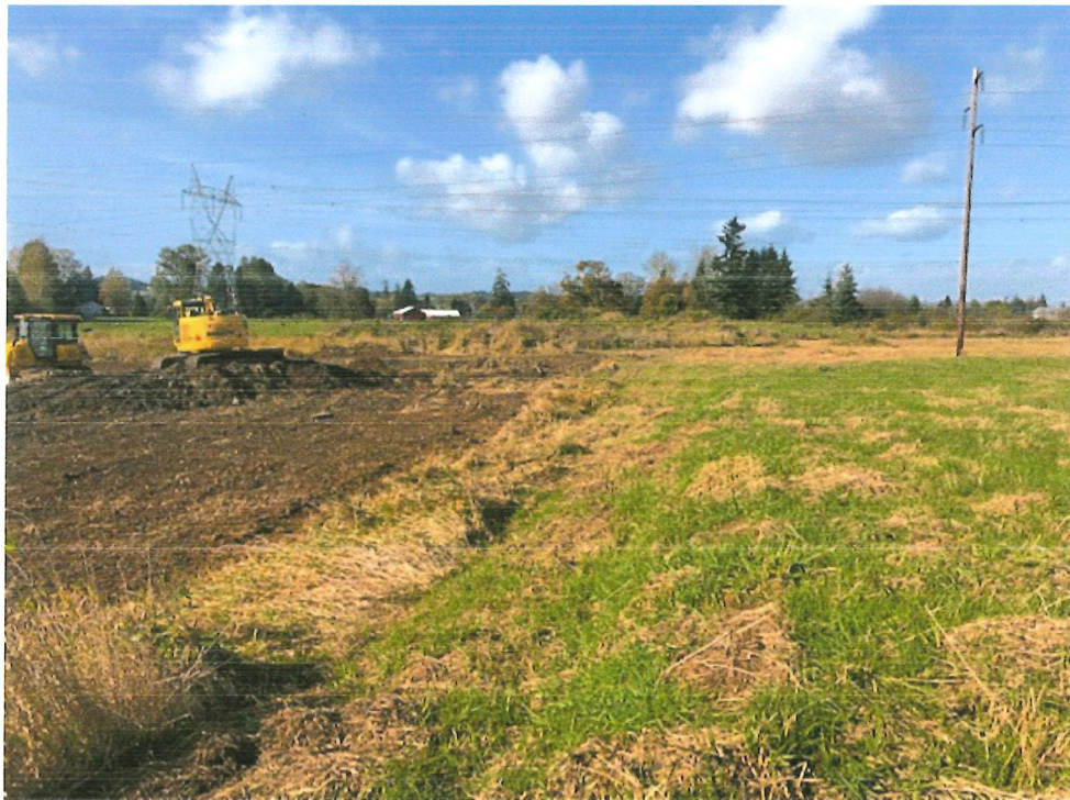
North view along the west property line. There is not inlet or outlet to this in defined ditch.
