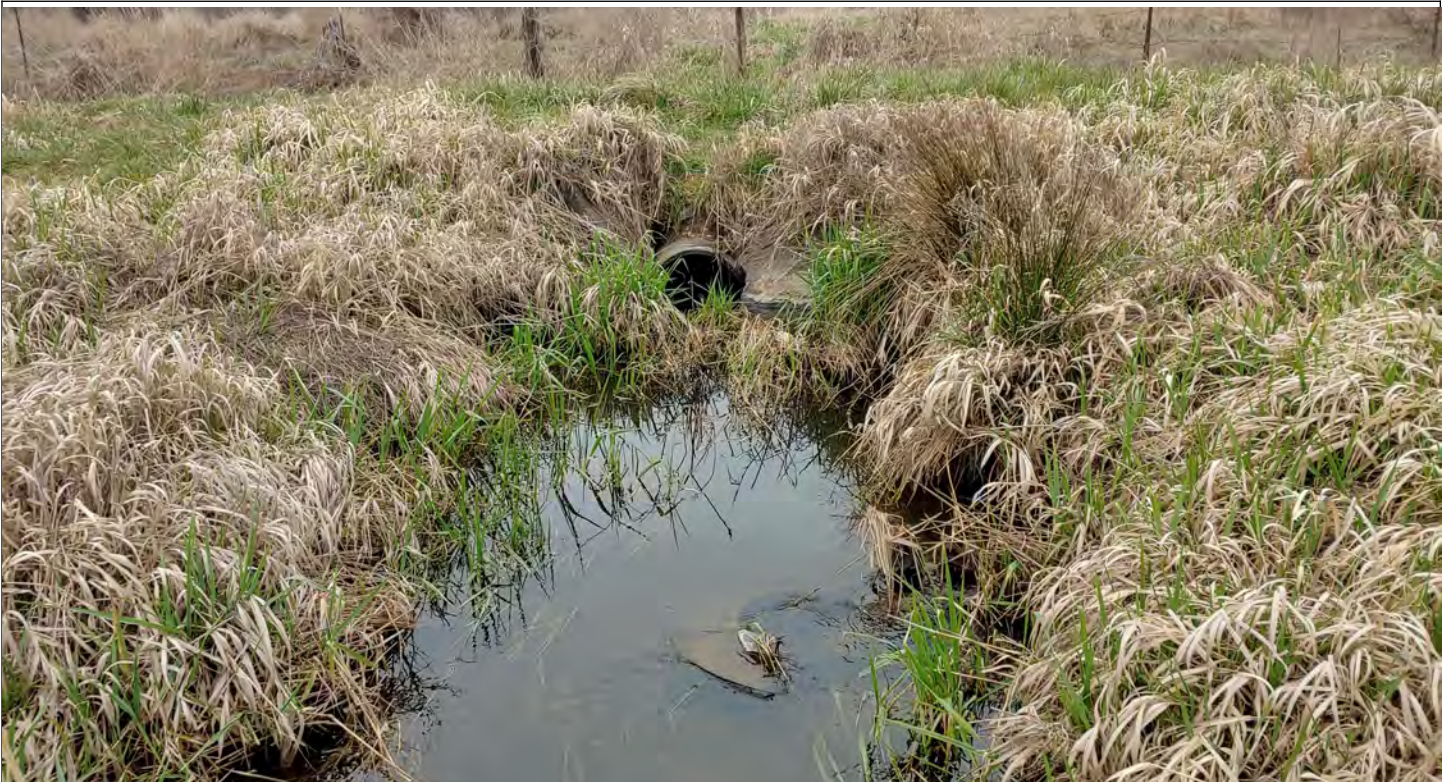
Above: (Photopoint 10) View east showing Ditch A and crossing with culvert, March 2019.
