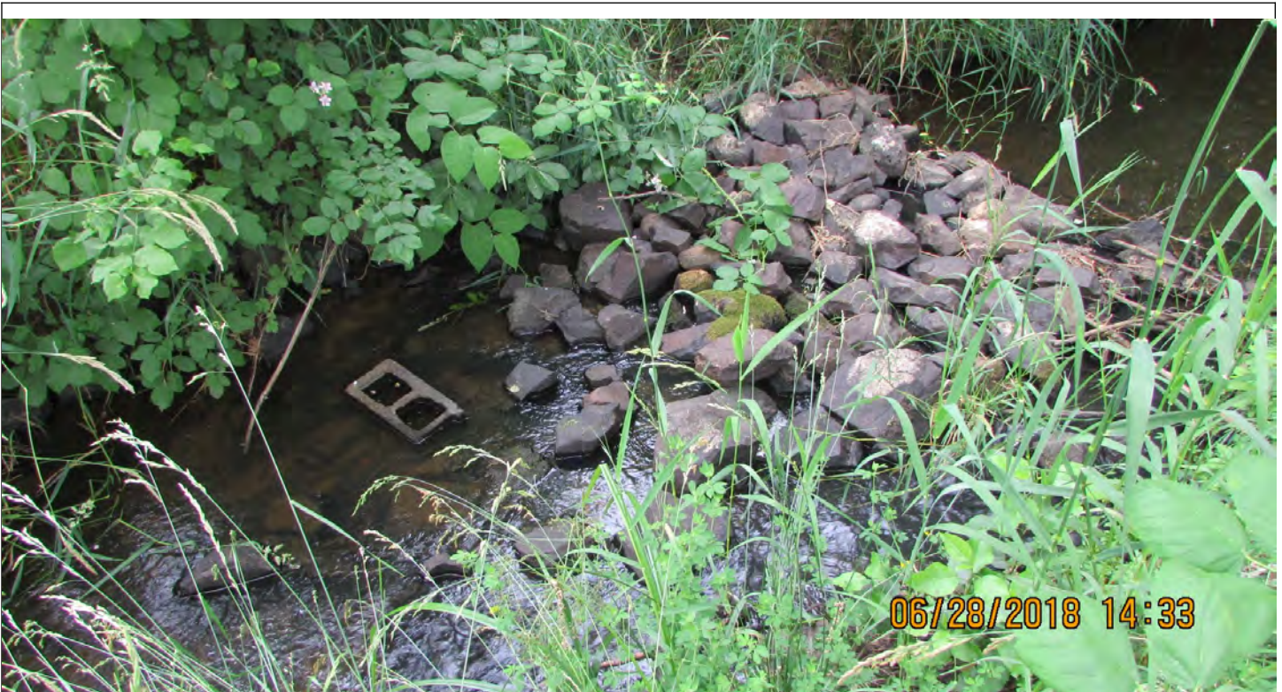
Above: (Photopoint 2) rock "dam" and other debris clogging Bewick Creek's channel.
