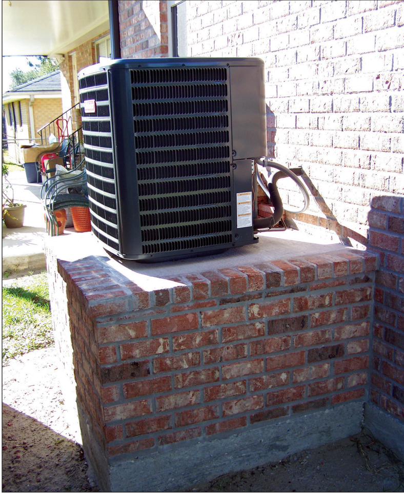
Figure 9-1. Air conditioning / heat pump compressor mounted on a brick pedestal outside an elevated home.
